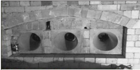
Refractory lining and burner blocks without coating
